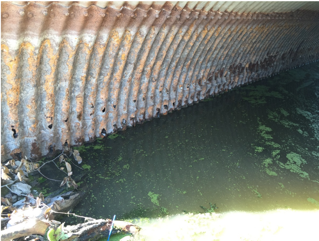
Typical Culvert Deterioration at Waterline
