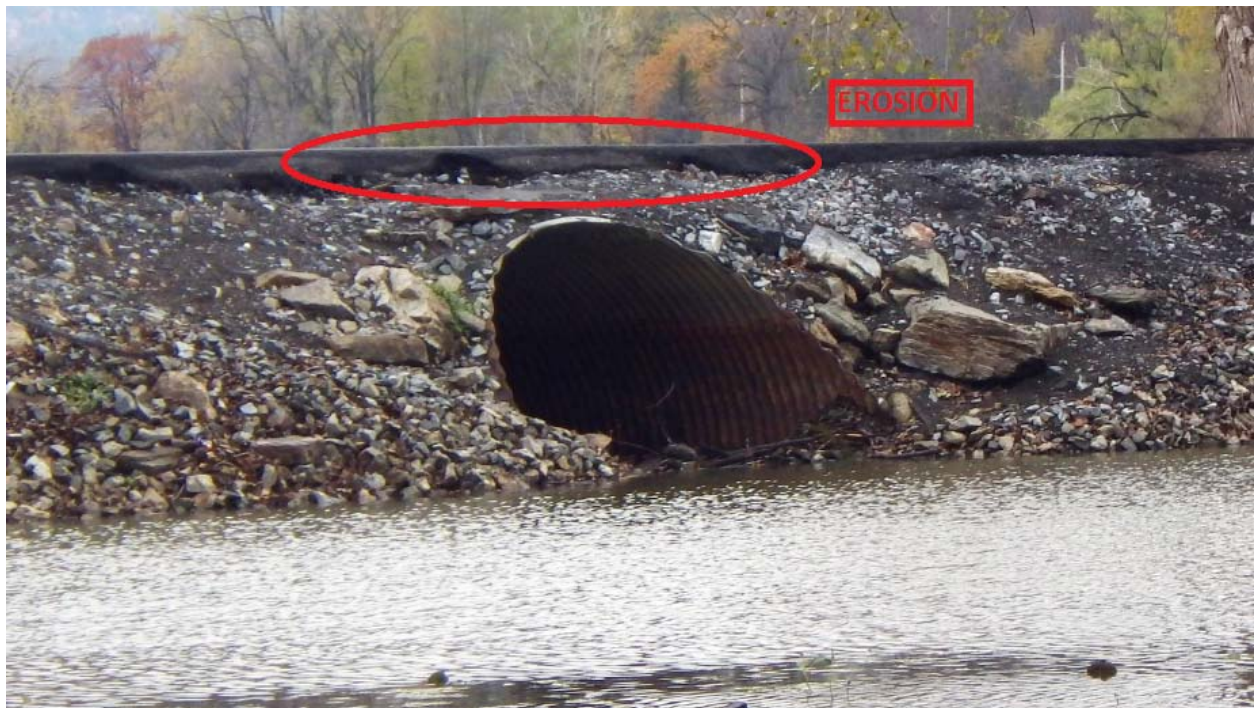
Figure 2: Erosion on the Bank above the Inlet
