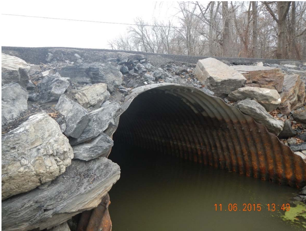
Figure 5: Large Stone Surrounding Culvert Outlet and Erosion above the Culvert
