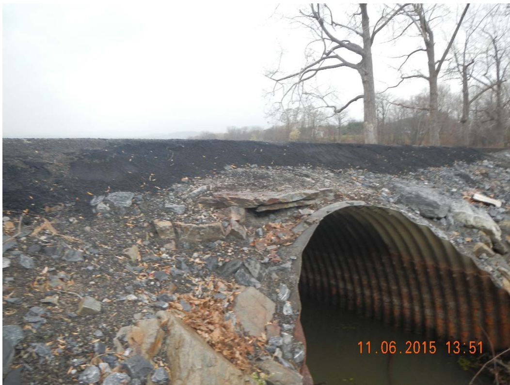
Figure 6: Large Stone Partially Surrounding the Culvert Inlet
