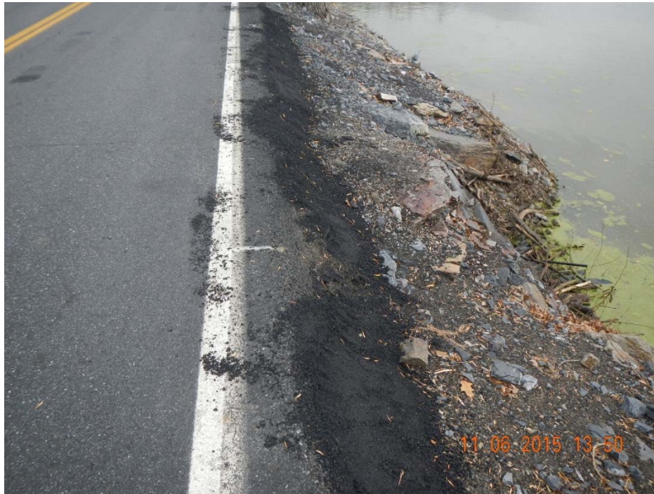
Figure 7: Shoulder Rehab for Erosion Located above the Culvert Inlet
